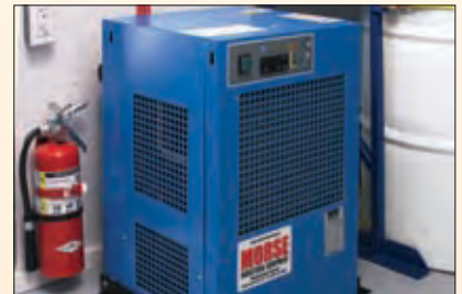
Air dryer keeps humidity levels down within the air supply system
